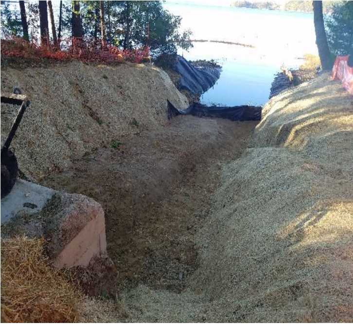
Fig 5: Sediment controls on the east side of the Bay at the Beswick property. Viewing west. (10-21-19).
