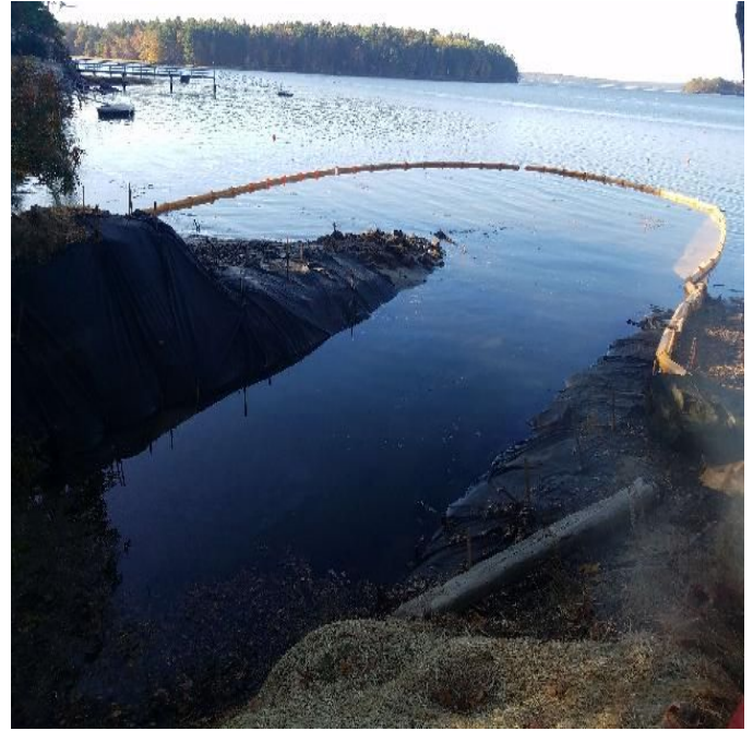
Fig 6: Silt curtain installed on the east side of the Bay. Viewing west. (10-21-19).
