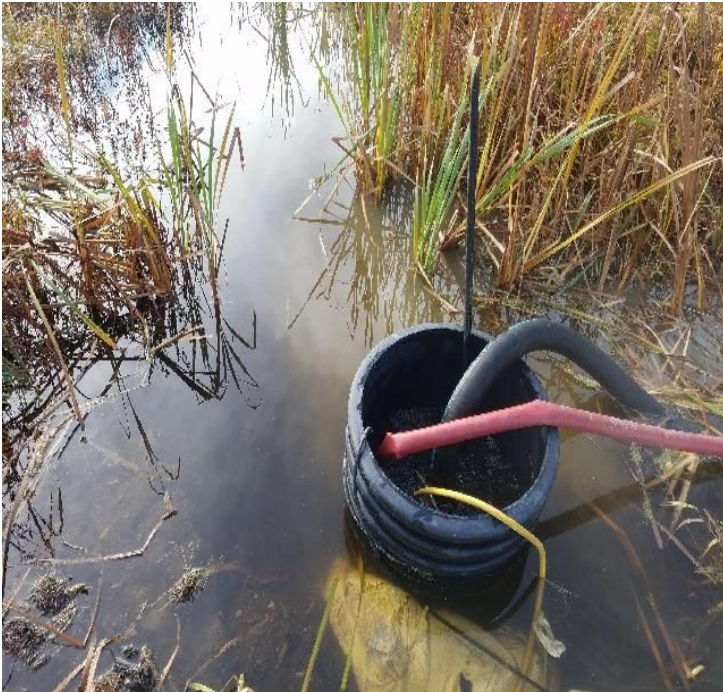
Fig 17: Turbidity visible around stream bypass pump in Knights Brook. Viewing south. (10-23-19).
