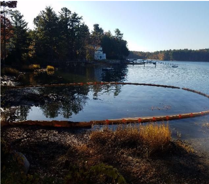
Fig 7: Silt curtain installed on the east side of the Bay. Viewing west. (10-21-19).
