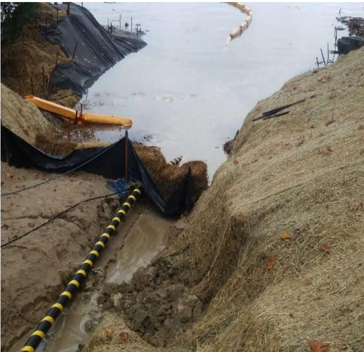
Fig 15: Trench walls washed out at Beswick Property. Viewing west. (10-23-19).
