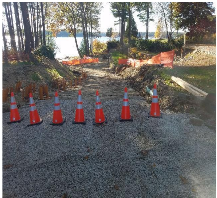
Fig 4: Access to man hole on the east side of the Bay at the Beswick property. Viewing west. (10-21-19).
