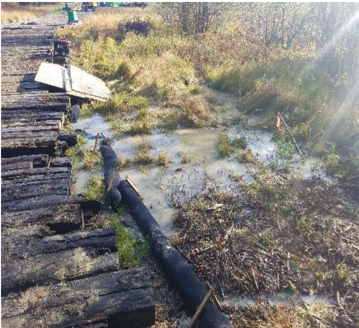
Fig 19: Turbid water, a result of the rutting near Str. 106. Viewing east. (10-23-19).
