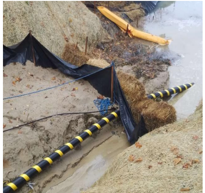
Fig 14: BMP failure around cable location. Viewing southwest. (10-23-19).
