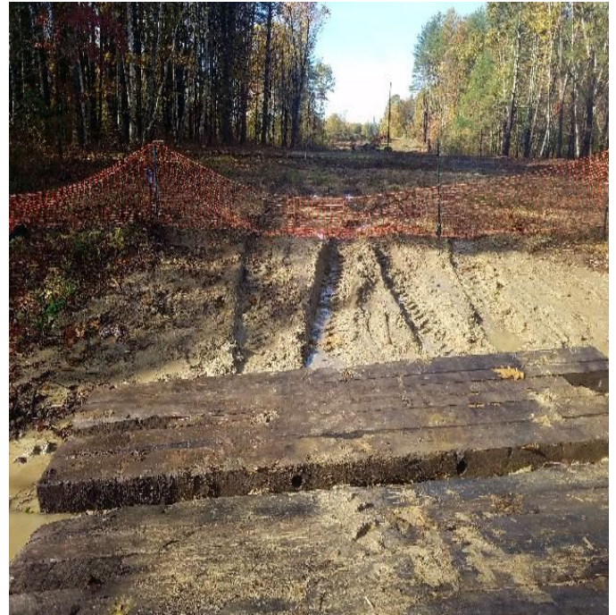
18: Ruts in previously restored area near Str. 106 causing sediment loss. Viewing west. (10-23-19).
