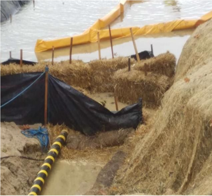
Fig 21: Temporary repairs made to sediment and erosion controls at Beswick property. Viewing west. (10-23-19).
