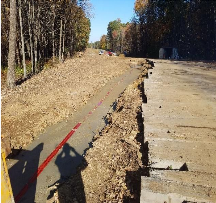
Fig 3: Float fill poured on duct bank in trench at Str. 107. Viewing west. (10-21-19).
