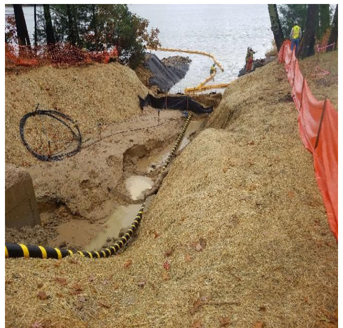
Fig 20: LS Cable and Blu Rock on site to patch sediment and erosion Controls at Beswick Property. Viewing west. (10-23-19).
