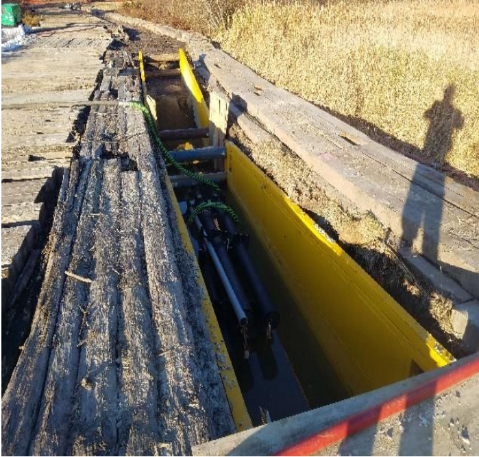
Fig 1: Pumping water out of trench and into frack tank at Frink farm. Viewing east. (10-21-19).
