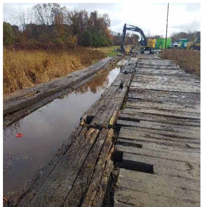
Fig 16: Approximately 1.5ft of water on top of float fill in trench at Frink farm. Viewing east. (10-23-19).
